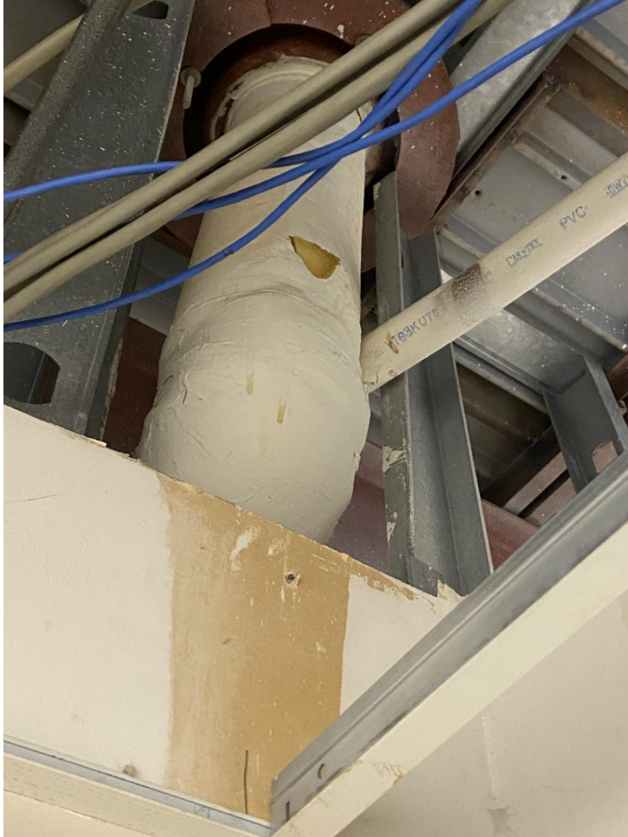
Asbestos-Containing Roof Drain Mastic Insulation 3% Chrysotile Inside Building
