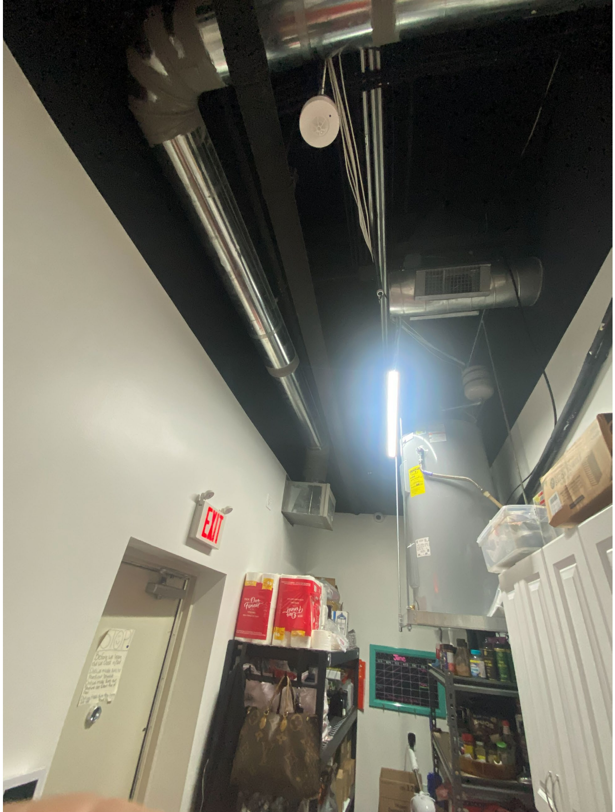
Plumbing at tenant space below GameDay
